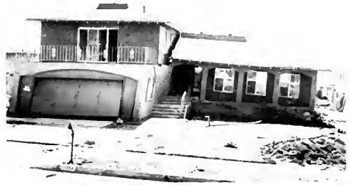
Photo 23. The one-story unit of this house settled and moved to the right following failure of the vertical (cripple) bracing between the floor and the footings. Courtesy of the City of Los Angeles Department of Building and Safety.
